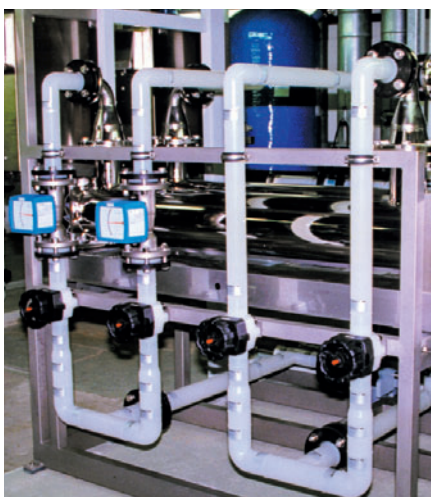
DI water treatment
