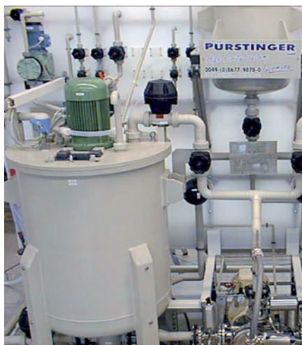
Slurry supply (company Puerstinger)
