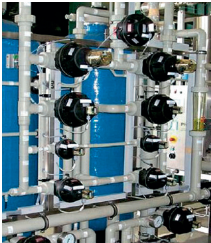
Plant with PP components
