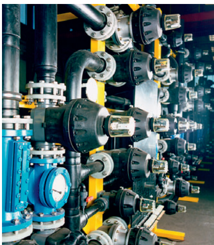
Waste water plant with PVC/PE components
