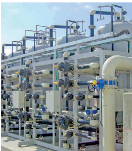
Water treatment (company Treitel Chemical Engineering Ltd)
