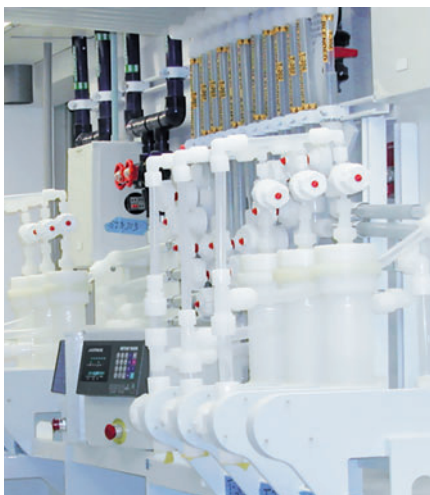
Chemical filling installation
